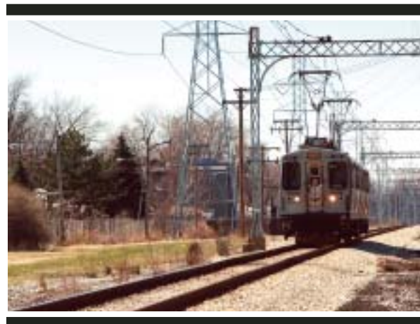
Catenary lines powering the Yellow Line will soon be replaced by contact rail.
