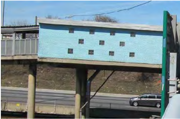
View of cracked and spalled concrete at base of stationhouse wall
