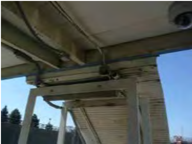
View of corrosion and peeling paint at platform canopy and walkway canopy at west end of station
