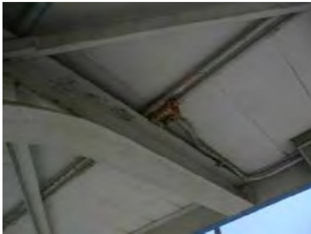
View of peeling paint and rusting conduit and junction box at platform canopy structure
