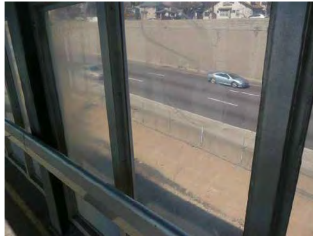
View of scratched and corroded surface of wind break enclosure at ramp
