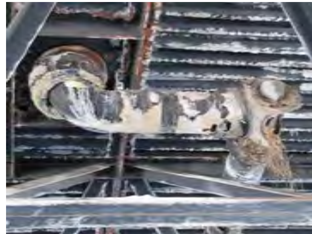
View of corroded roof drain with birds nest at platform level canopy
