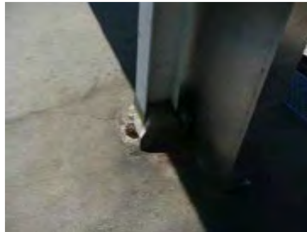
View of broken concrete at base of platform canopy columns.
