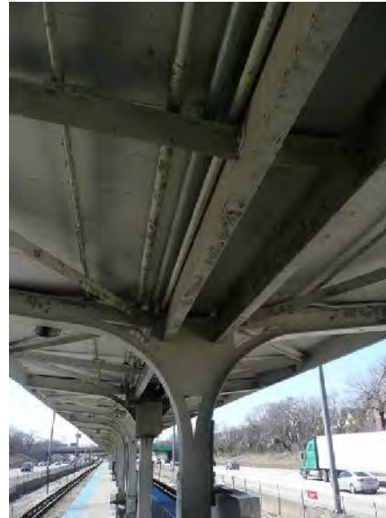
View of peeling paint at platform canopy structure
