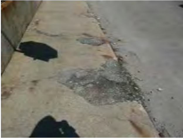
View of broken and patched sidewalk along East Avenue near stationhouse entry
