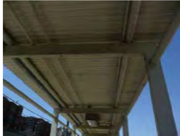
View of peeling paint at walkway canopy near East Avenue platform entry
