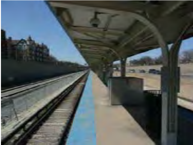
View of non-compliant platform with impeding elements
