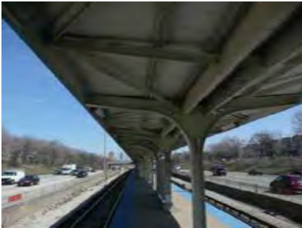
View of peeling paint and rusting at platform canopy structure
