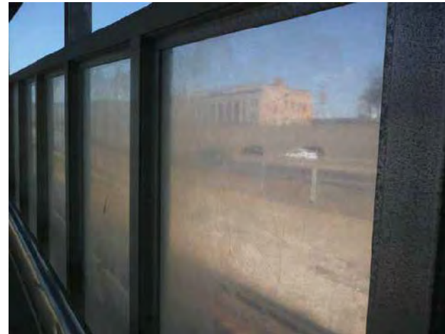
View of aged plastic panels and corroded aluminum surface of wind break enclosure at ramp
