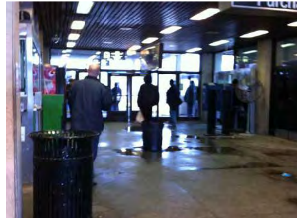
View of roof drains leaking through ceiling at unpaid area
