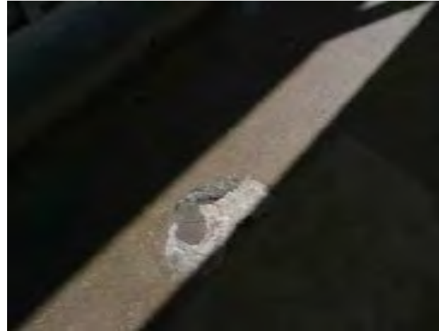
View of broken concrete and patch at ramp surface
