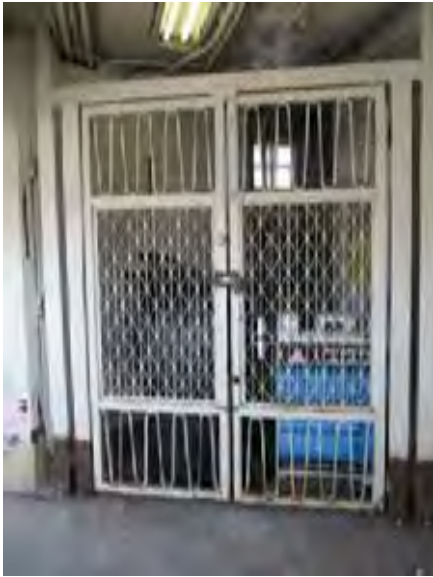
View of corrosion and deterioration at base of gates and main stationhouse
