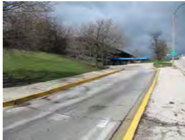
View of inclined sidewalk at north side approach to station. Note sidewalk is likely too steep to meet ADA slope requirements.
