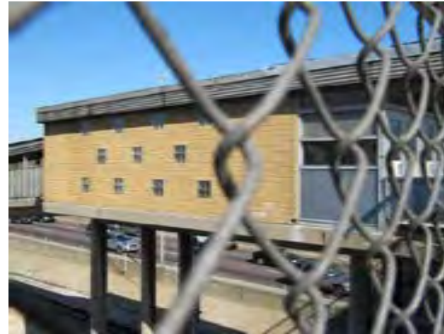
View of Harlem Stationhouse showing roof edge condition, brick condition and evidence of water infiltration to rebar within concrete.
