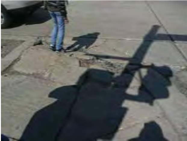
View of crosswalk and curb ramp at Cicero and Flournoy intersection. Note broken sidewalk curb ramp that should be repaired.
