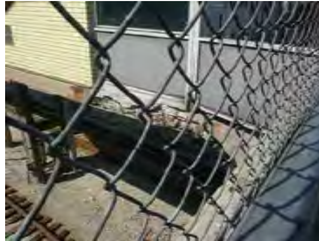
View of cracked and spalled concrete at base of stationhouse wall. Note re-bar is exposed and deterioration is advanced.
