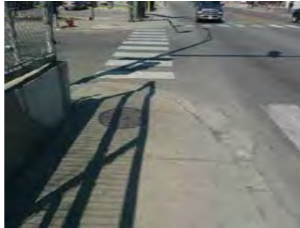
View of sidewalk condition along Pulaski near Congress Note broken sidewalk and portions of curbs that should be repaired.
