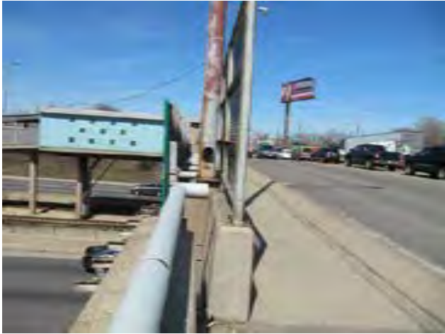
View of corrosion and open electrical junction box at light post on Cicero bridge overpass.
