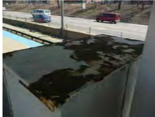
View of peeling paint and rusting at platform storage box elements.
