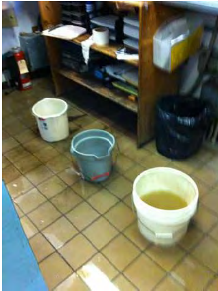
View of roof drains leaking through ceiling at customer service kiosk
