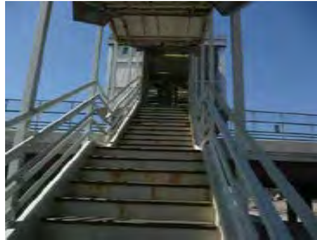
View of west exit stair showing rust at risers
