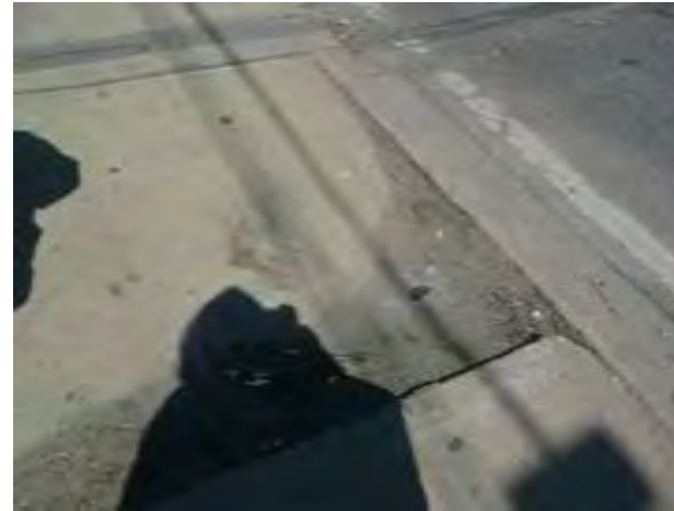
View of sidewalk condition along Cicero near Lexington. Note broken and sunken portion of sidewalk that should be repaired.
