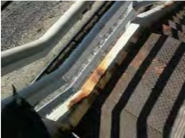
View of rusting structure at stair near East Avenue entry
