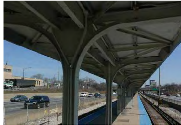
View of non-compliant platform with impeding elements
