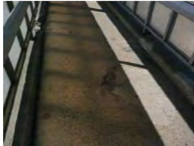
View of broken concrete at ramp walking surface. Note also broken concrete curb at wind break
