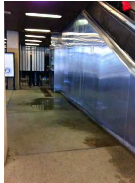
View of roof drains leaking at escalator enclosure down into paid area
