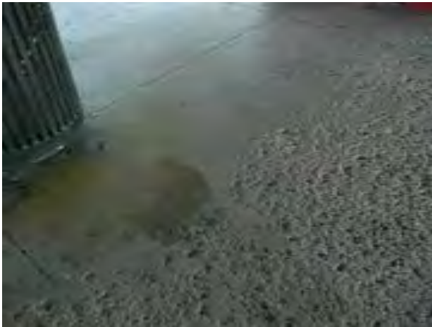
View of spalling concrete at platform surface
