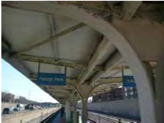
View of peeling paint and rusting conduit at platform canopy structure
