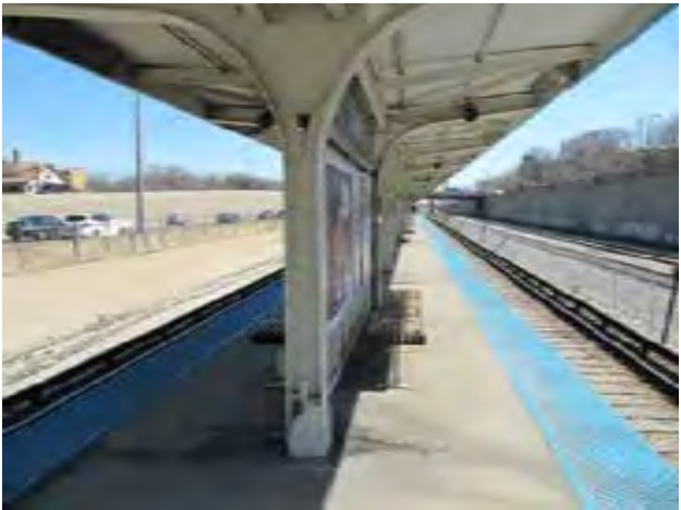
View of Austin Platform showing broken concrete near base of platform canopy columns
