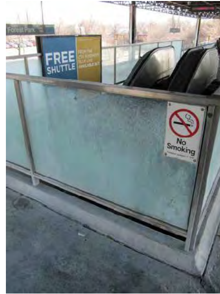
View of whitish surface deposits on guardrails, concrete and railings throughout the platform area.
