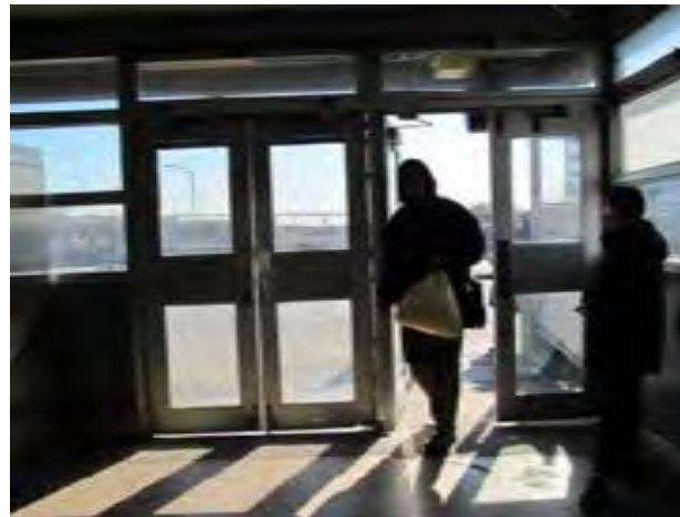
View of non-compliant entry doors at Harlem Avenue Station
