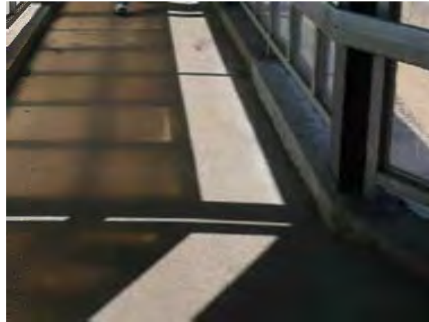
View of broken concrete and patching at ramp surface
