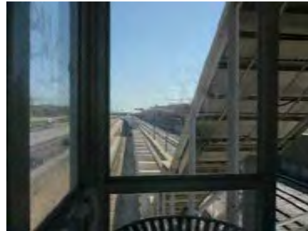
View of west stationhouse windbreak enclosure showing scratches and deterioration
