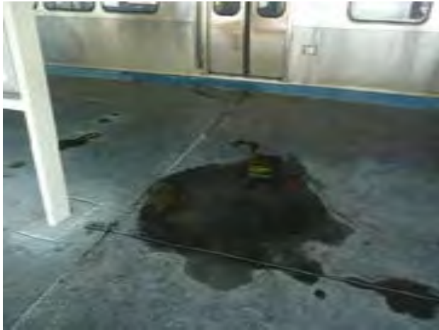
Evidence of roof drains leaking on platform level
