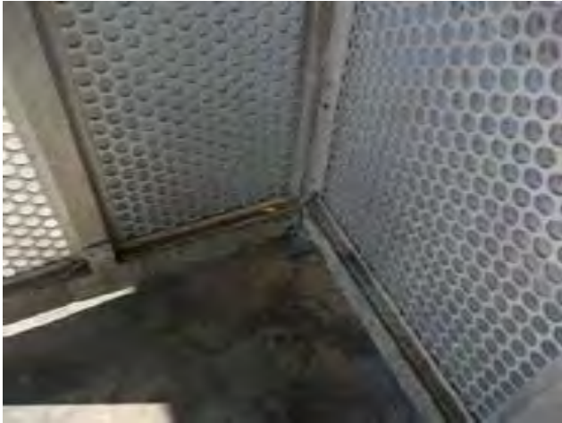
View of corrosion at windbreaks on platform
