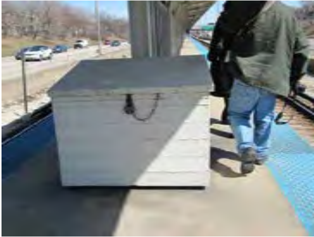
View of non-compliant platform with impeding elements
