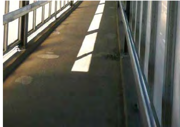
View of broken concrete and patch at ramp surface
