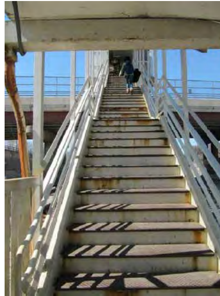
View of exit stair and at west end of walkway from platform
