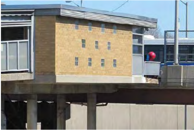
View of Austin Stationhouse showing deterioration and spalling at concrete near guardrail
