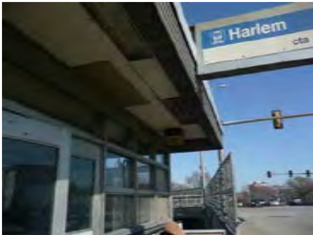
View of missing light diffusers and panels at roof eave at main station entry
