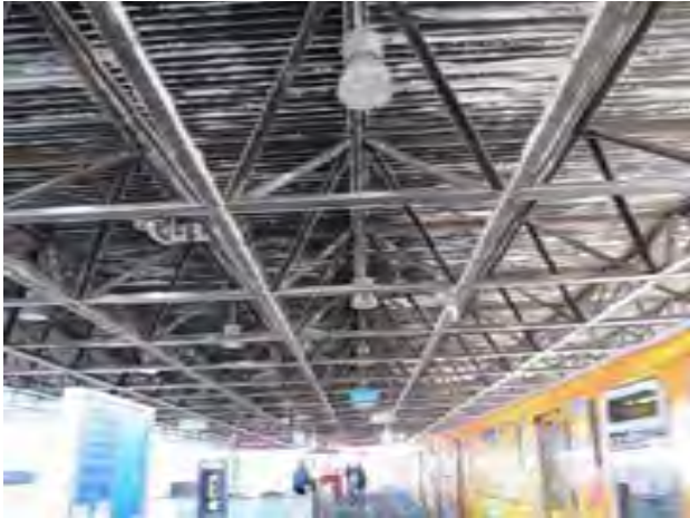
View of peeling paint and rusting components at platform canopy structure
