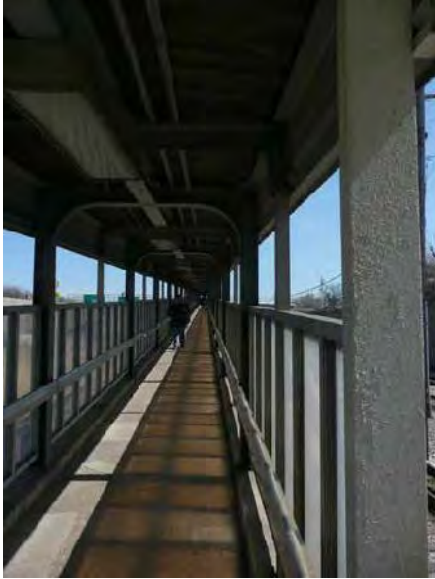
View of non-compliant ramp from platform to station house
