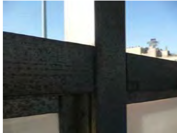
View of corroded surface of wind break enclosure at ramp
