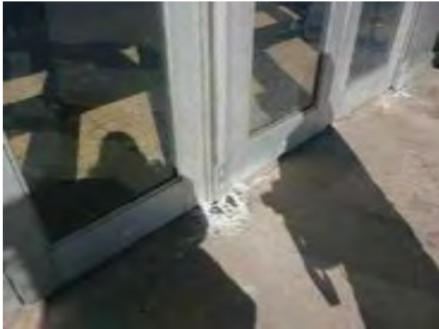
View of corrosion and deterioration at base of main entry doors
