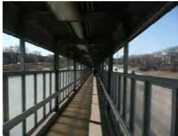
View of non-compliant ramp from platform to station house
