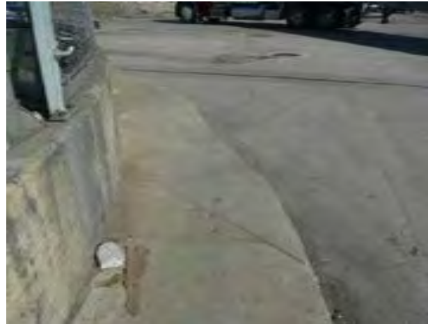
View of non-compliant curb ramp at Harlem Avenue on approach to station. Note that the pedestrian crosswalk is not identified with striping
