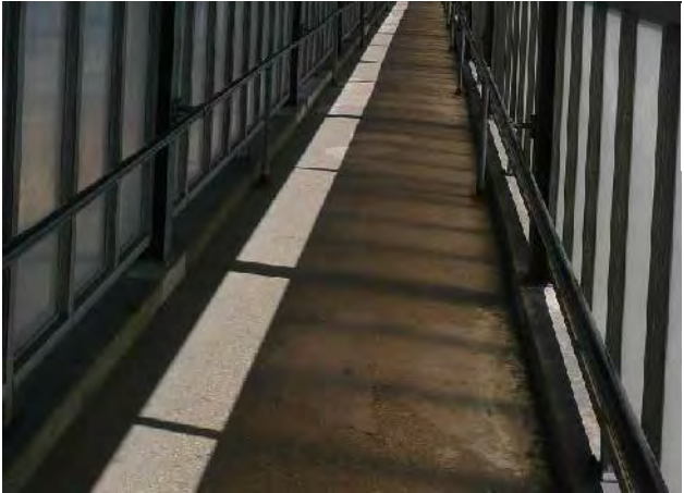
View of broken concrete and patches at ramp surface. Note rusting at base of handrail support posts.
