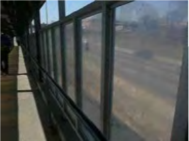
View of corrosion and aged, scratched surface of wind break enclosure panels at ramp
