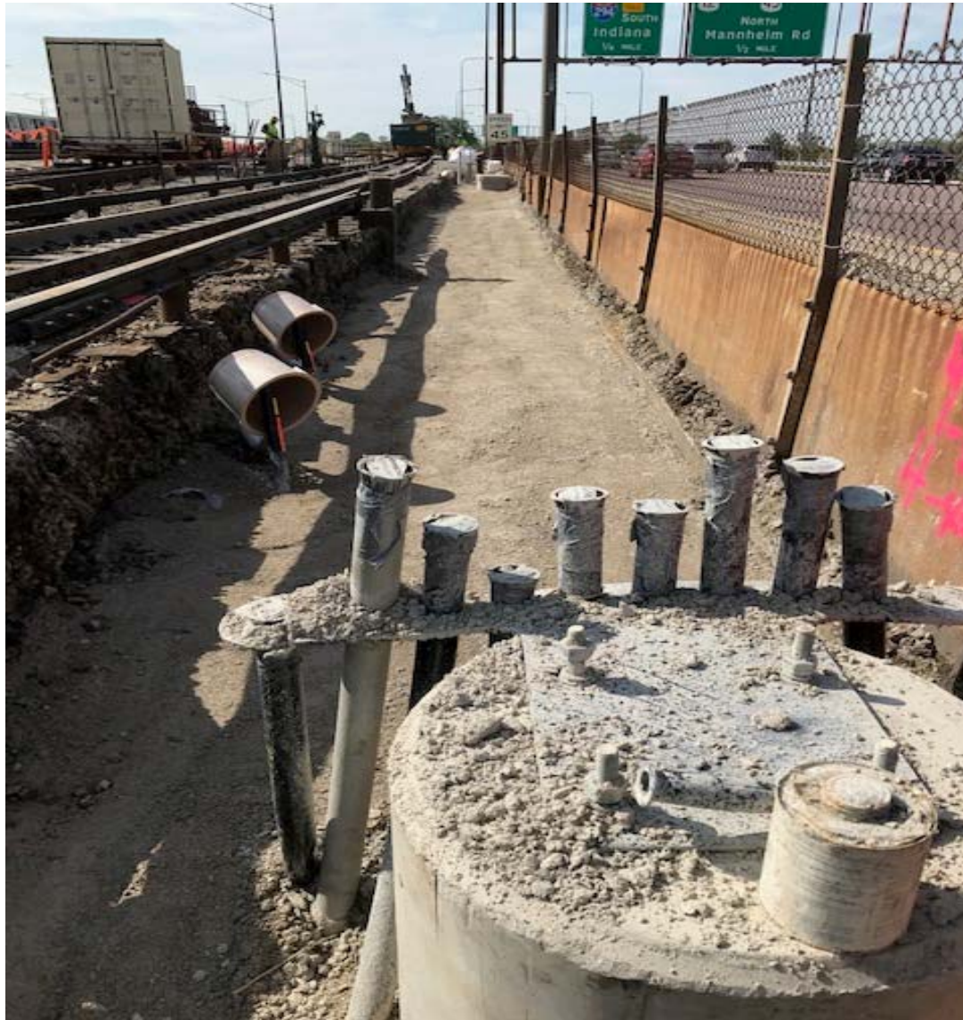
Underground Infrastructure for Switch Heat
