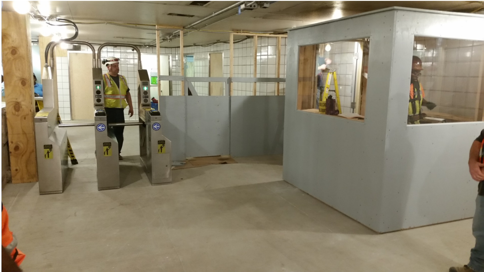
Transition of Mezzanine Work at Chicago Station Temporary Kiosk and Fare Equipment Installation
