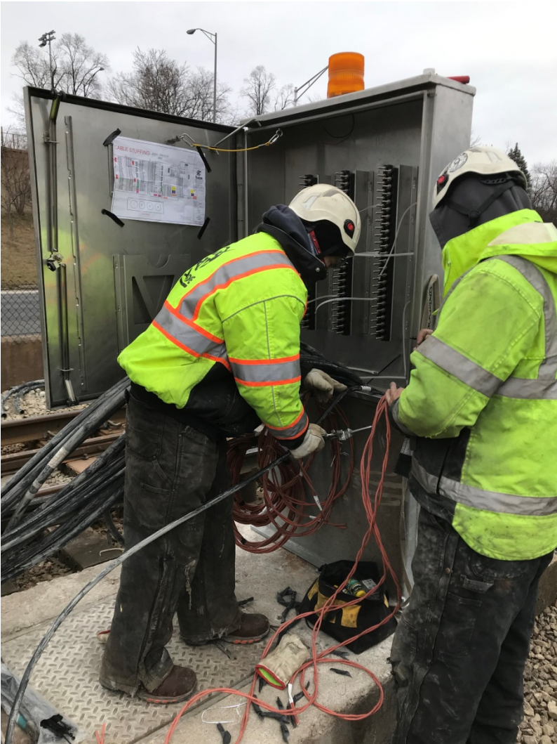
Junction Box Wiring at Nagle Interlocking
