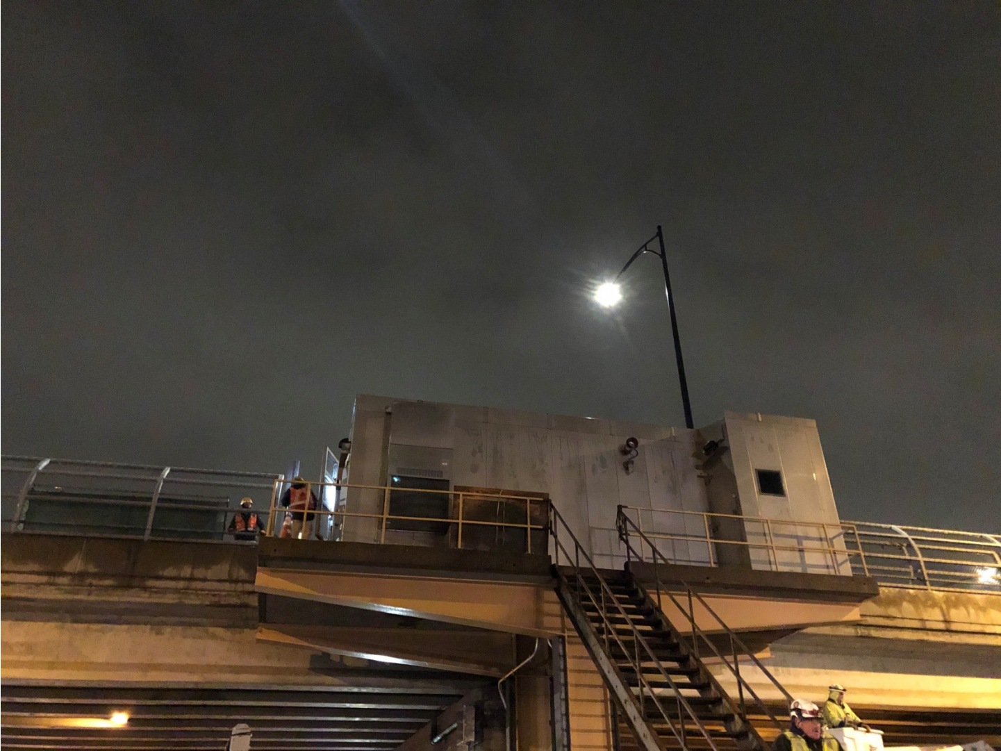
Nagle Relay House Installation
