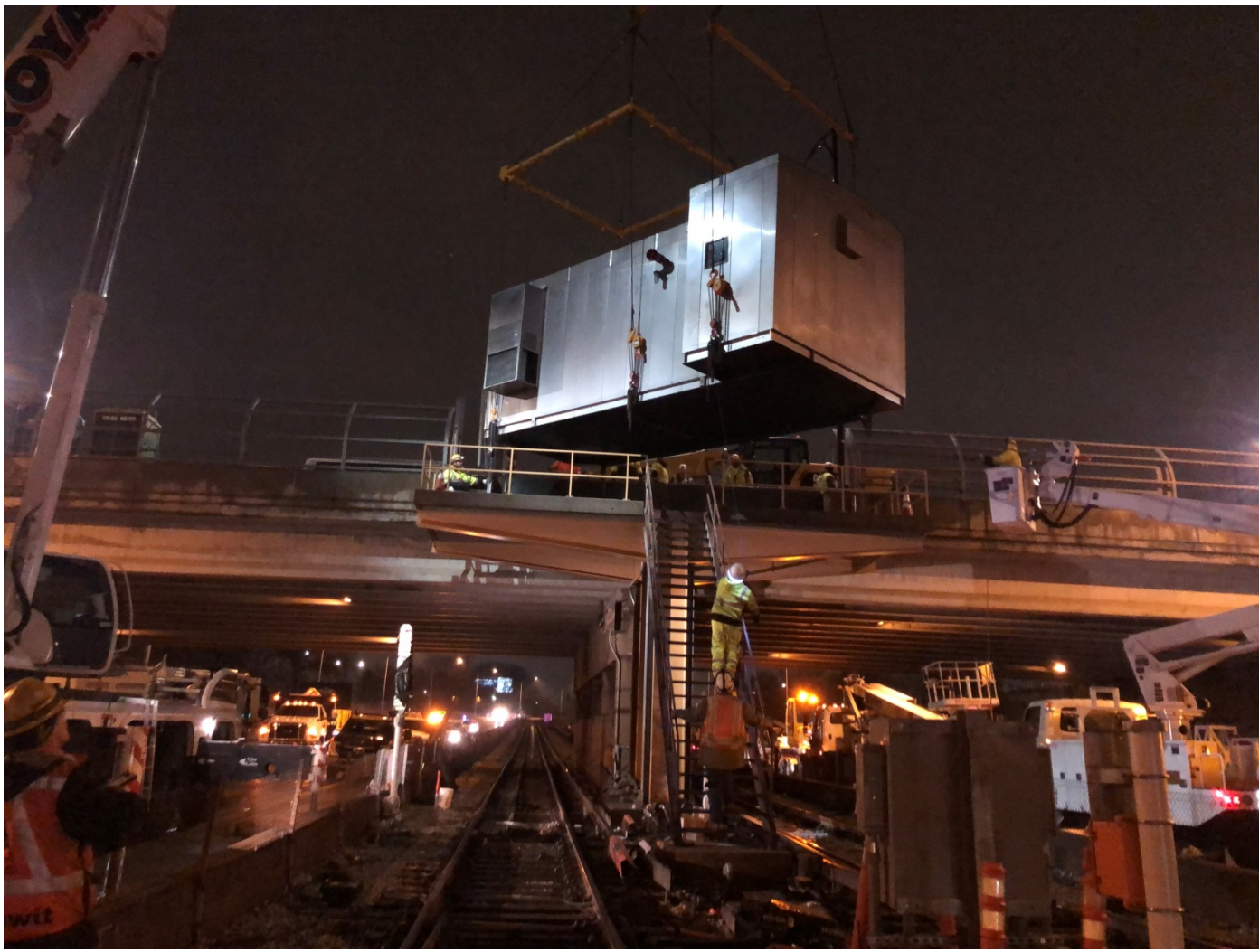
Nagle Relay House Installation
