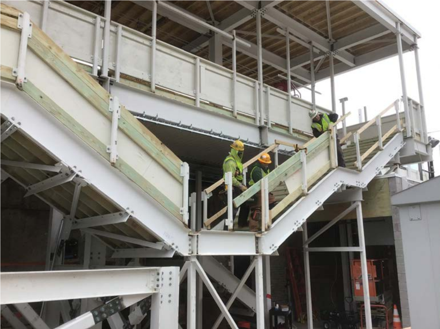
LBMM - Argyle Temporary Station
