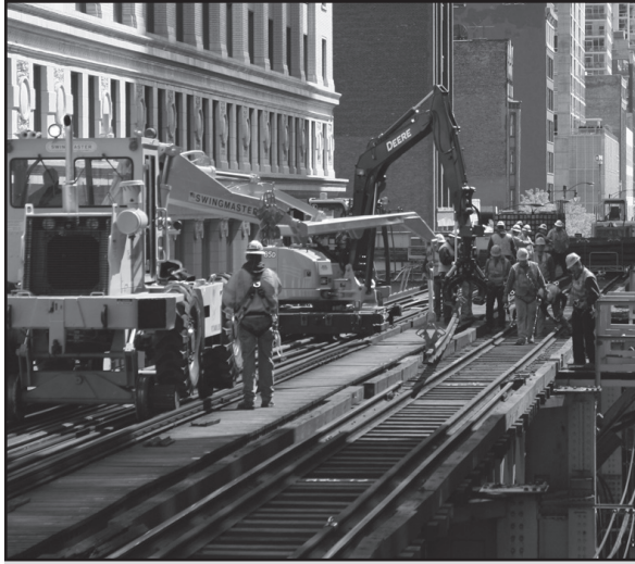
CTA's Loop Track Renewal project was one of the agency's largest construction projects in 2012 and was on schedule to be completed by year-end. The $33.8 million project replaces more than two miles of elevated rail and track components that were installed in the early 1980s and are nearing the end of their useful life.
