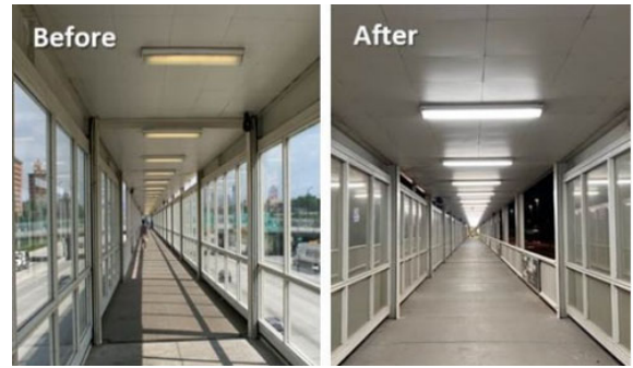
Lighting upgrade in the pedway at the Sox-35 th Red Line Station
