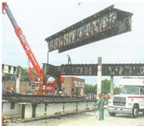
With matching funds from the State of Illinois, CTA was able to rebuild the 54th/Cermak branch of the Blue Line.
