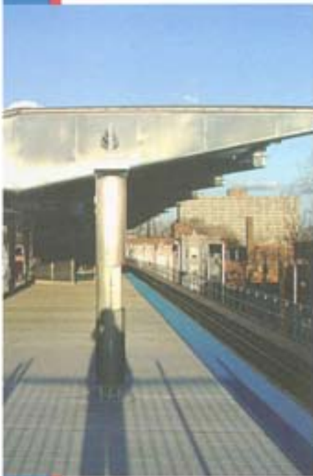
The renovated platform at the Kedzie station on the 54th/Cermak branch of the Blue Line features a stainless steel canopy.
