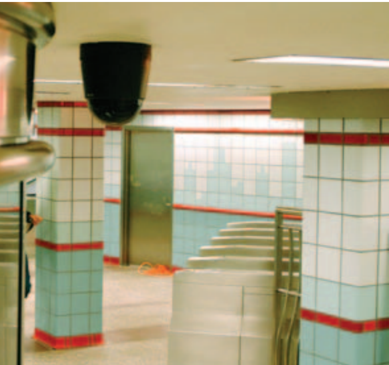
Security cameras, such as the one pictured here on the Red Line Lake station mezzanine, are part of CTA's ongoing effort to enhance security on its system.
