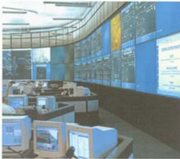
CTA's Control Center constantly monitors trains and buses in service throughout the area.
