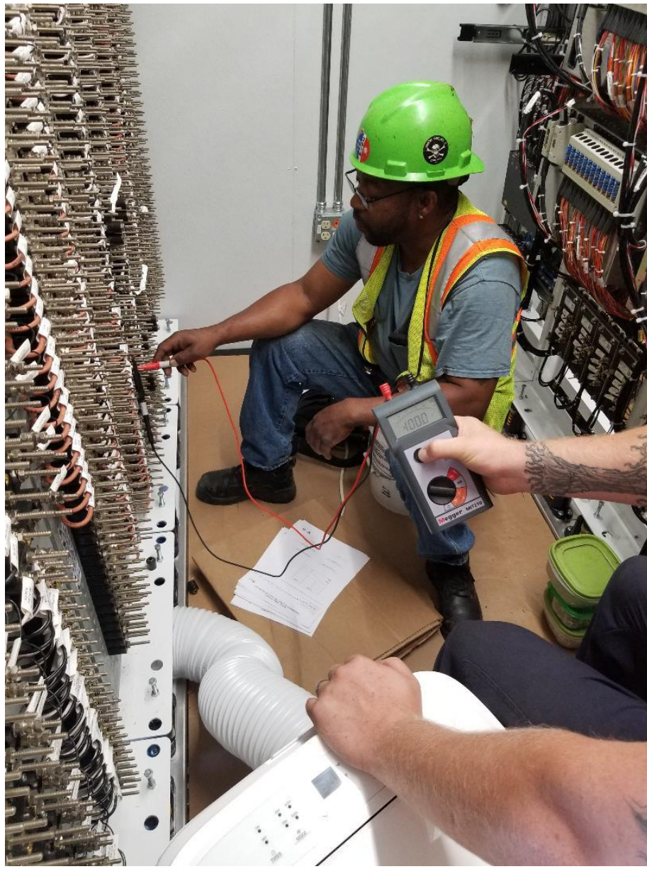
Megger Testing of Relay House Equipment
