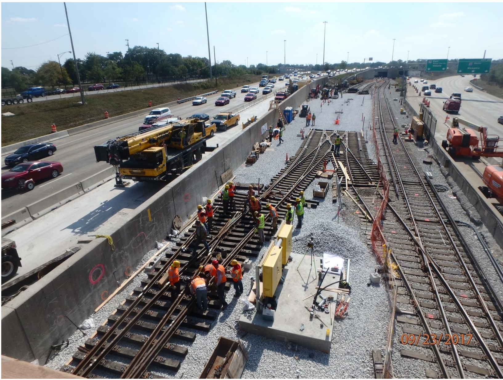
96 th Interlocking Installation
