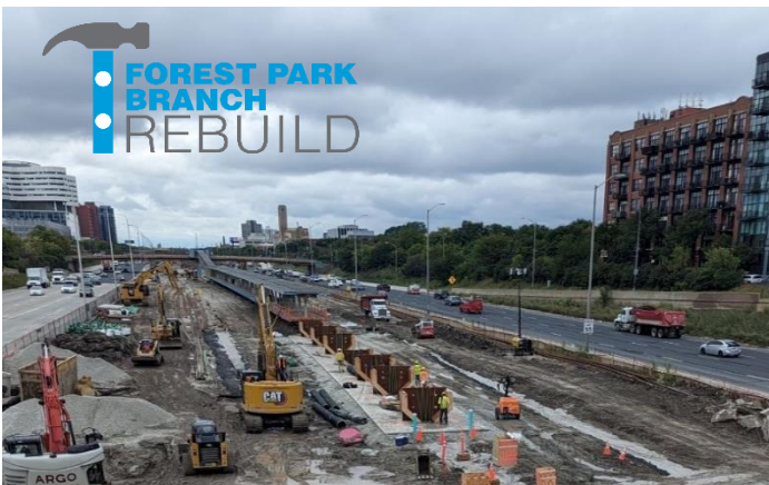
Under Phase 1 of the Forest Park Branch Rebuild, crews completely removed and rebuilt nearly three miles of track bed along the Blue Line branch. Work also includes upgrading the power and signal systems and completely reconstructing the Racine station.
