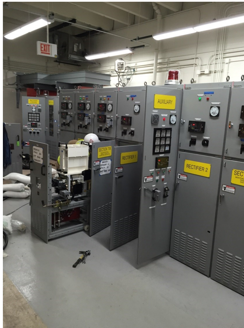
Kimball Substation: New Traction Power Equipment Installed
